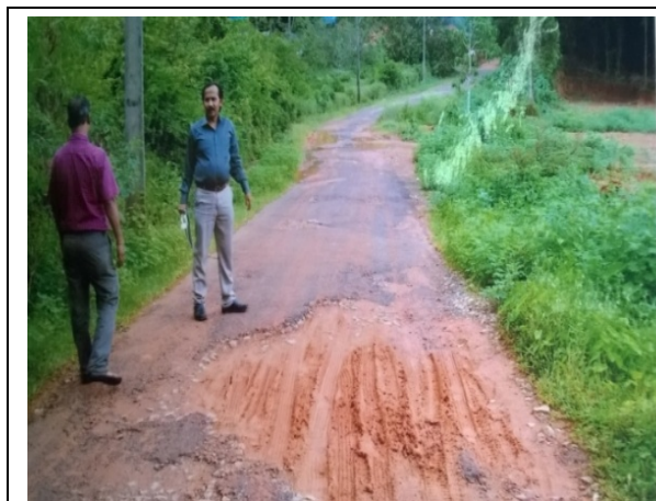
Condition of asphalted road within six months of construction in Aivathoklu village (Dakshina Kannada) (16.07.2014)
